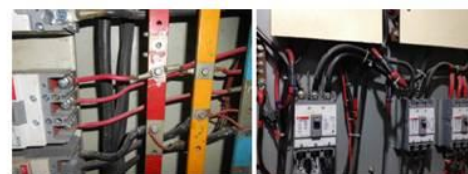
Outer insulation damaged in live electrical wires
